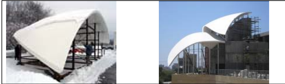
Figure 13 manufacturing the roof using GRP and foam blocks of polystyrene as a mould Architect Moshe Safdie. 2003-2005
