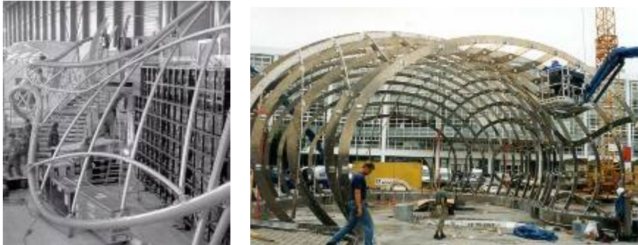
Figure 10 BMW pavilion, designed by Bernhard Franken, 2000, Source: Kolarevic, Branko, Architecture in the digital age, 2005
