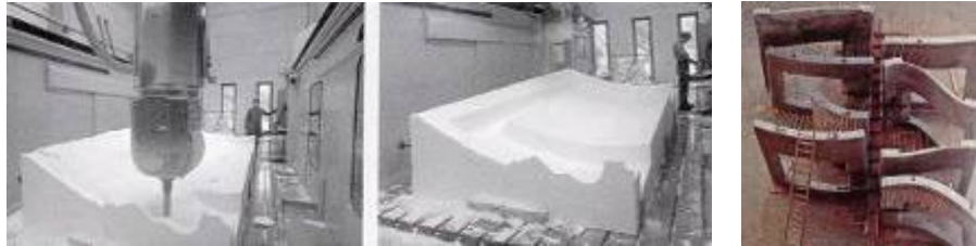
Figure 6 The CNC multi-axis milled Styrofoam molds, which are fitted and in site assembled Source: Rempen ,Thomas, der Neue Zollhof Düsseldorf , Germany, 1999
